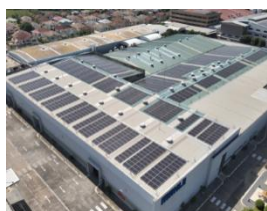
The photovoltaic installation at MAHLE Siam Filter Systems provides 1 MWp of installed solar capacity, generating more than 1100 MWh of renewable electricity each year.
