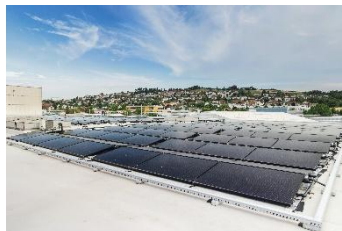
Around 780 of the more than 1,000 PVT modules are located on the roof of the main building at the MAHLE site in Vaihingen an der Enz.
